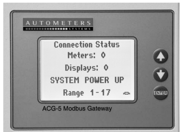
2. System Power up
